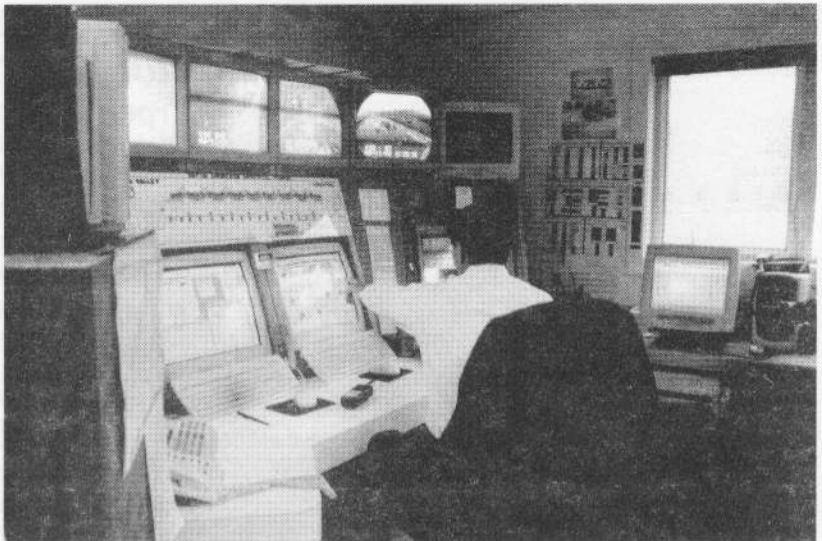
Control room for monitoring the Whittier Tunnel where trains and vehicles share the tunnel
